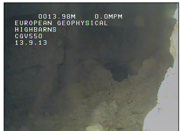
Void found in garden of 12 Highbarns
