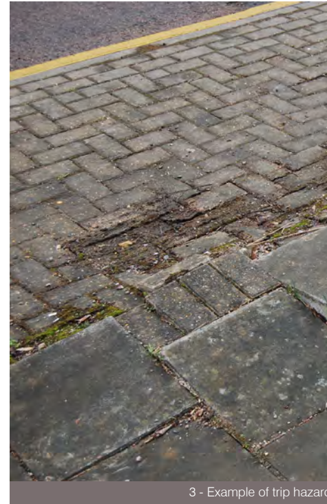
2 - Example of rutted pavement
